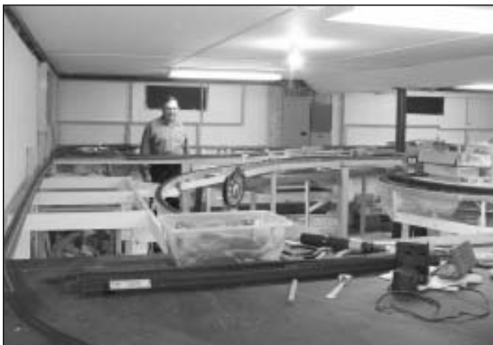
A panoramic view showing new ceiling and backdrop framing installed on the walls of the layout room.
